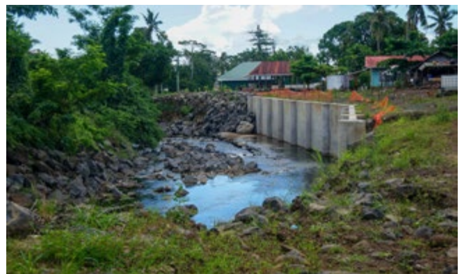
Flood protection near Malia’s home. The Green Climate Fund is supporting work to benefit 27,000 people living in the flood-prone Vaisigano river catchment in Apia, Samoa.
